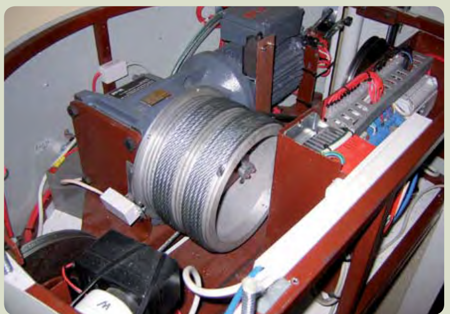
The pulley system of the lift.
